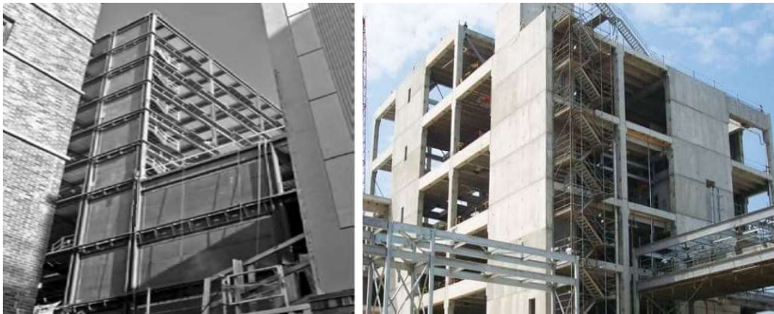
Fig. (1-1) : Location and shape of the steel plate and RC shear walls.
