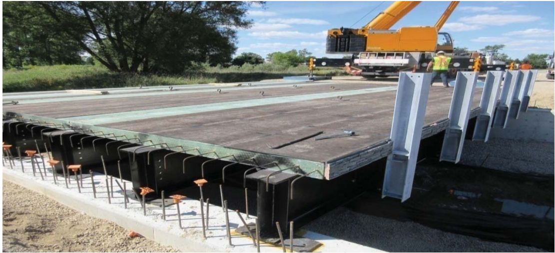
Figure (1-1) Using Composite Section in Bridge Construction (Guardian Bridge Rapid Construction Company) [21]
