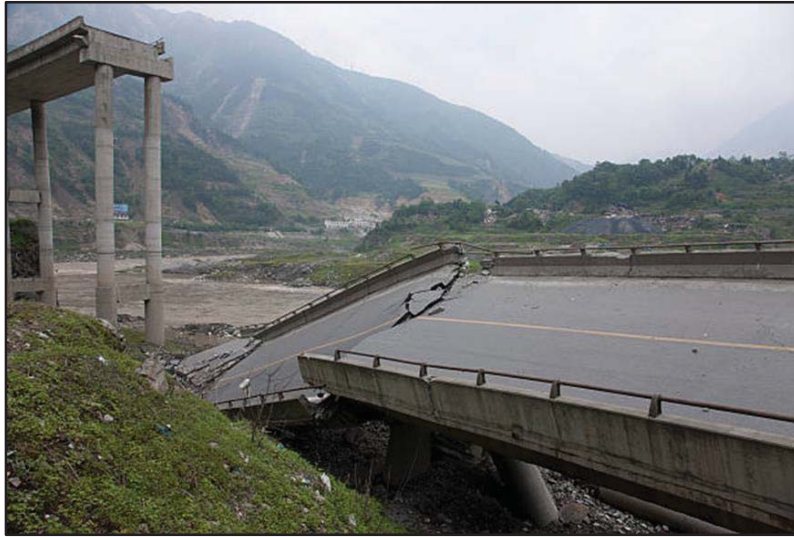
Figure (1.4): Collapsed of Kahramanmaraş Bridge in Turkey earthquake 2023 (National Earthquake Information Center).
