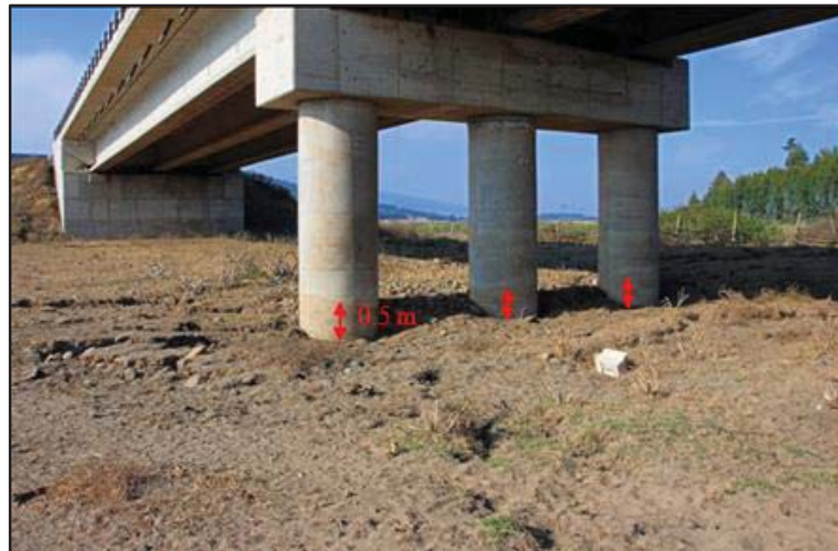
Figure (1.3): Soil settlement at interior pier at Mataquito Bridge (Gutierrez and Ledezma, 2017).
