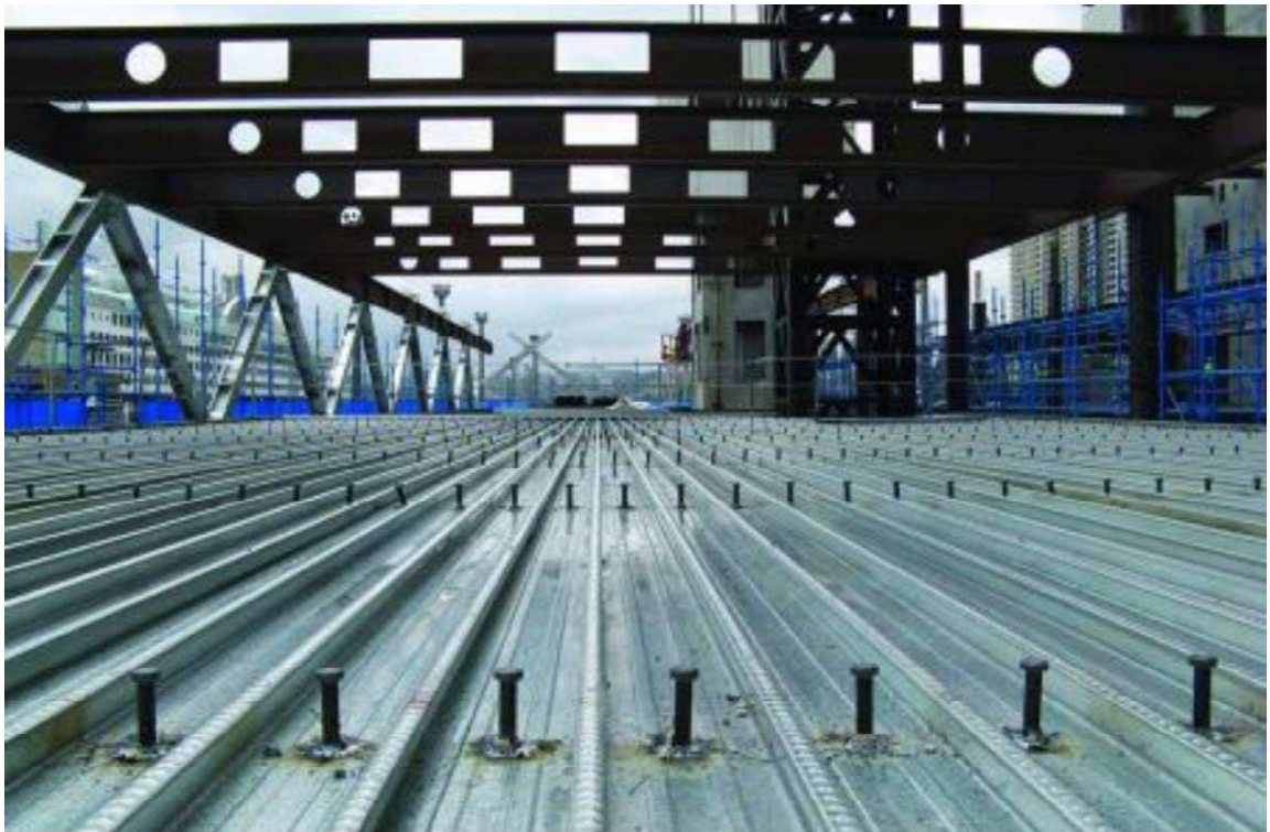
Figure (1-1) Composite Slab Construction, Showing the Steel Sheet Placed on Steel Frame (Lysaght)
