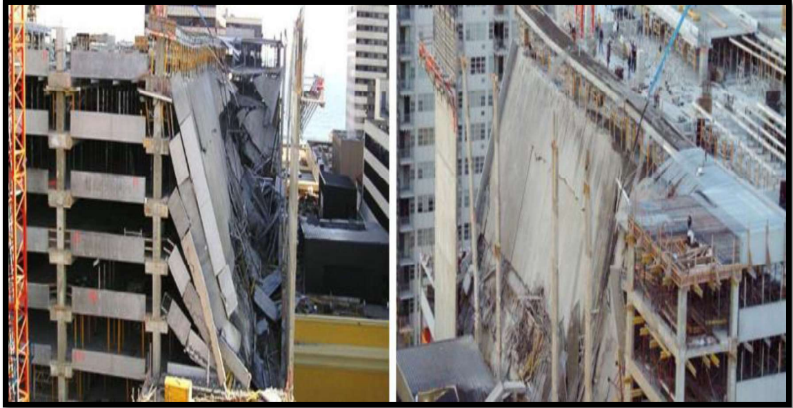
Plate (1-4): shear failure in beams of the parking garage in the Atlantic City (Bosela 2018)
