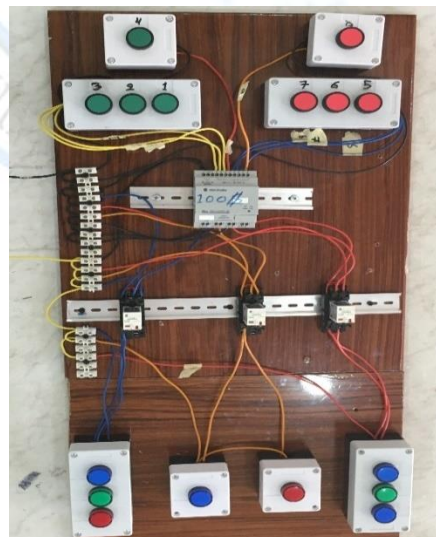
Fig.2 Electrical Control Panel
